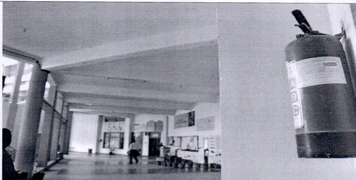
Maintaining Fire Safety Equipment throughout the campus in the VFSTR
