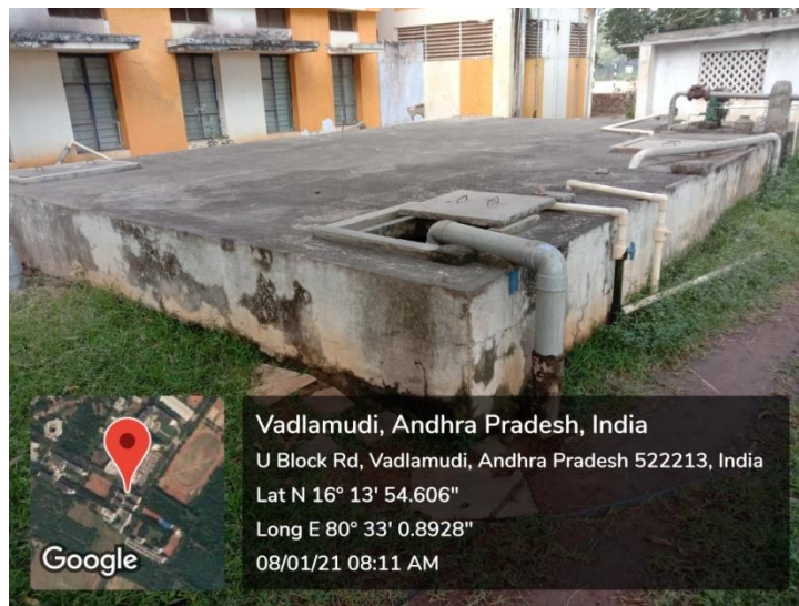
Fig 12. 58K Litres capacity tank at Vignan Vihar Boys Hostel
