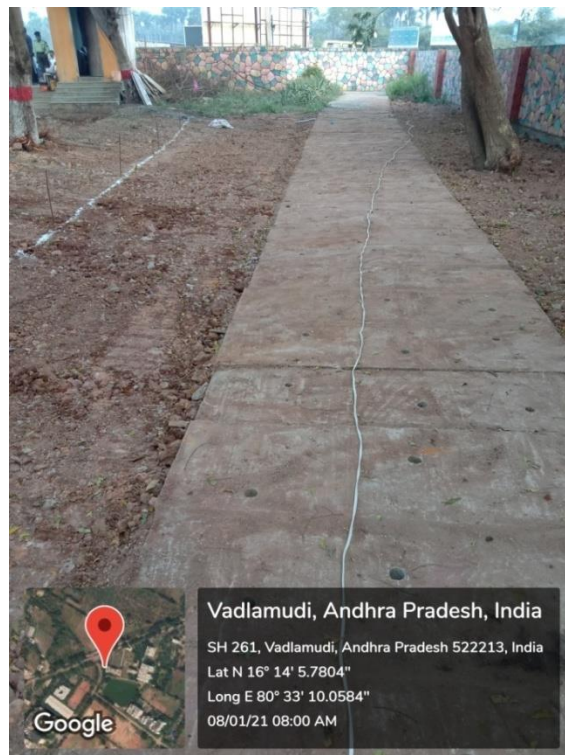
Fig 18. Closed Drain system at VFSTR campus
