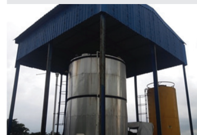
Image source: Biogas plant at VFSTR
